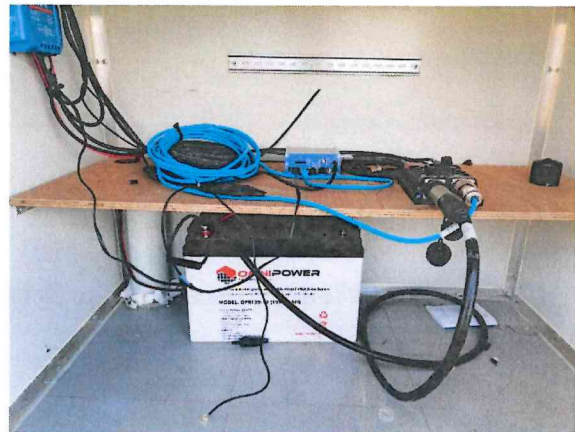
Figure 5: Inside the equipment housing
